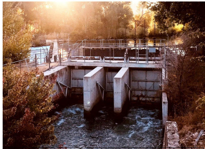
Workers will close these headgates at the head of the Ridenbaugh Canal near Barber Park the morning of Oct. 4 which will shut off all Boise River water flowing into the Nampa & Meridian Irrigation District’s canals. (NMID Photo)
